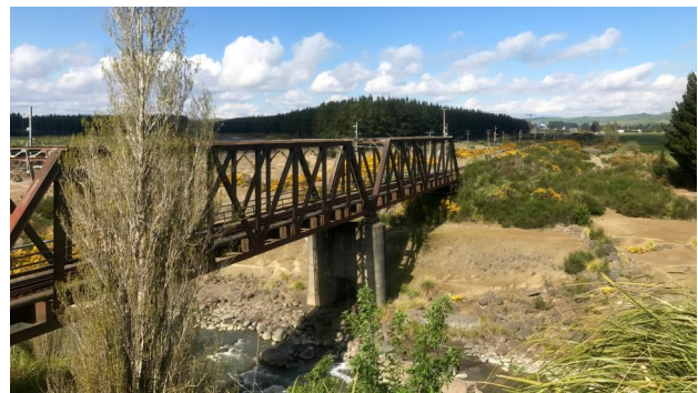
The new bridge built after the disaster still carries the North Island Main Trunk Railway across the Whangaehu River. The ill-fated express approached from the opposite bank.
